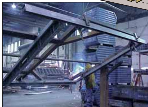
◀ Each frame is set-up and welded in a spinner jig for proper weld position to ensure the best possible weld penetration.
